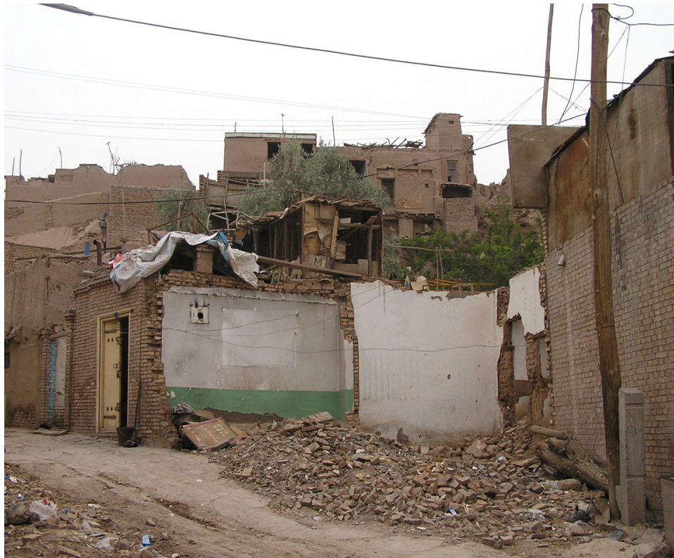
Houses in dilapidated state in old Kashgar (Photo by K.Warikoo)
